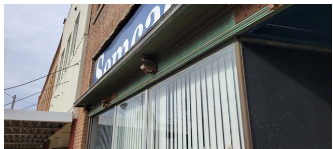
Top/Middle Top: Cornice/Parapet Conditions, 2024 (MacDonald & Mack Architects) Middle Bottom: Appropriate awning placement. Accessed 2024. (Google Earth) Bottom: Historic metal awning backband, 2023. (MacDonald & Mack Architects)
