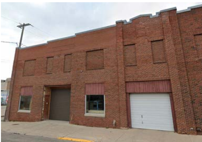
Top: Basement Entrance, 2023. (MacDonald & Mack Architects) Middle/Bottom: Historic building with overhead door openings on a primary facade. Accessed 2024. (Google Earth)
