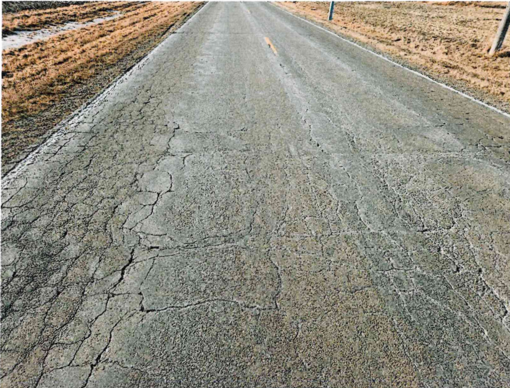
5 – SE Marshall St – Deteriorated Pavement
