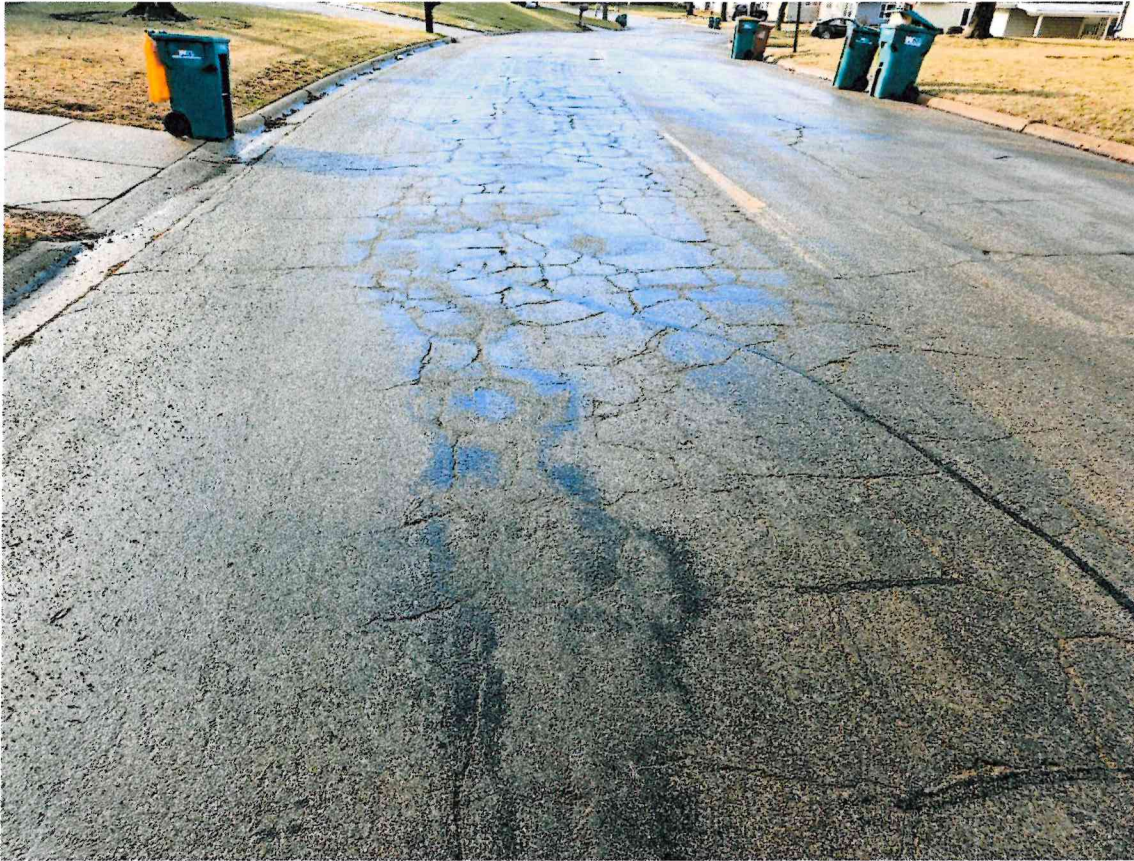
1 - Garfield Ave - Alligator Cracking
