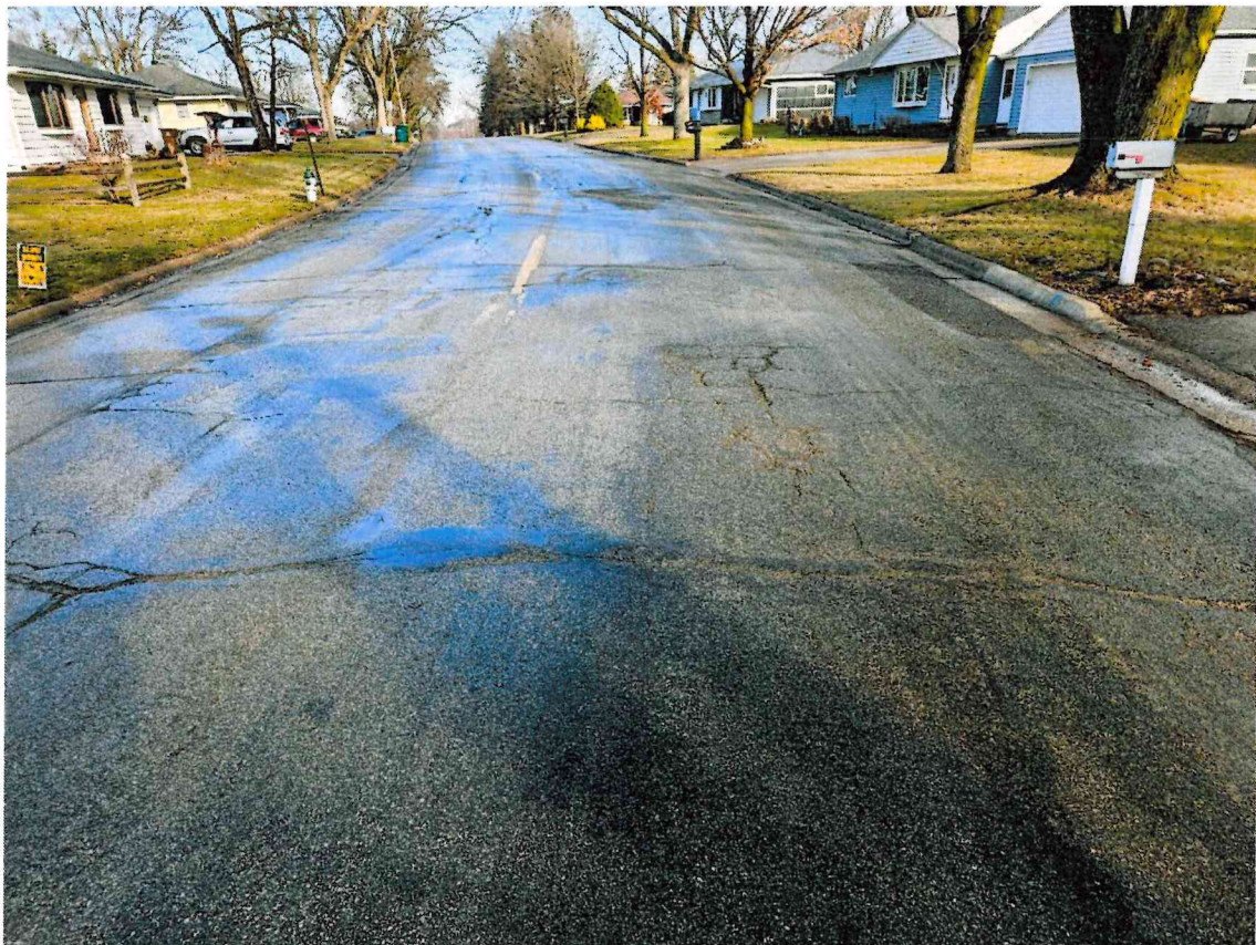
2 - Garfield Ave - Transverse & Longitudinal Cracking
