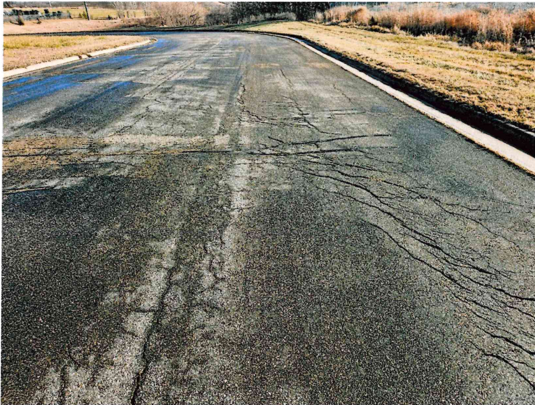
4 – Ross Drive – Deteriorated Pavement
