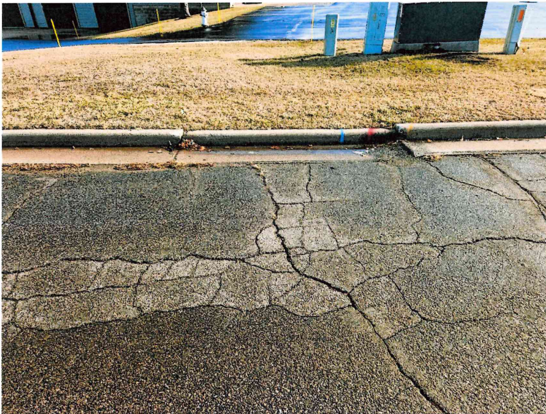
2 – Lake Chapeau Drive: Settled Curb
