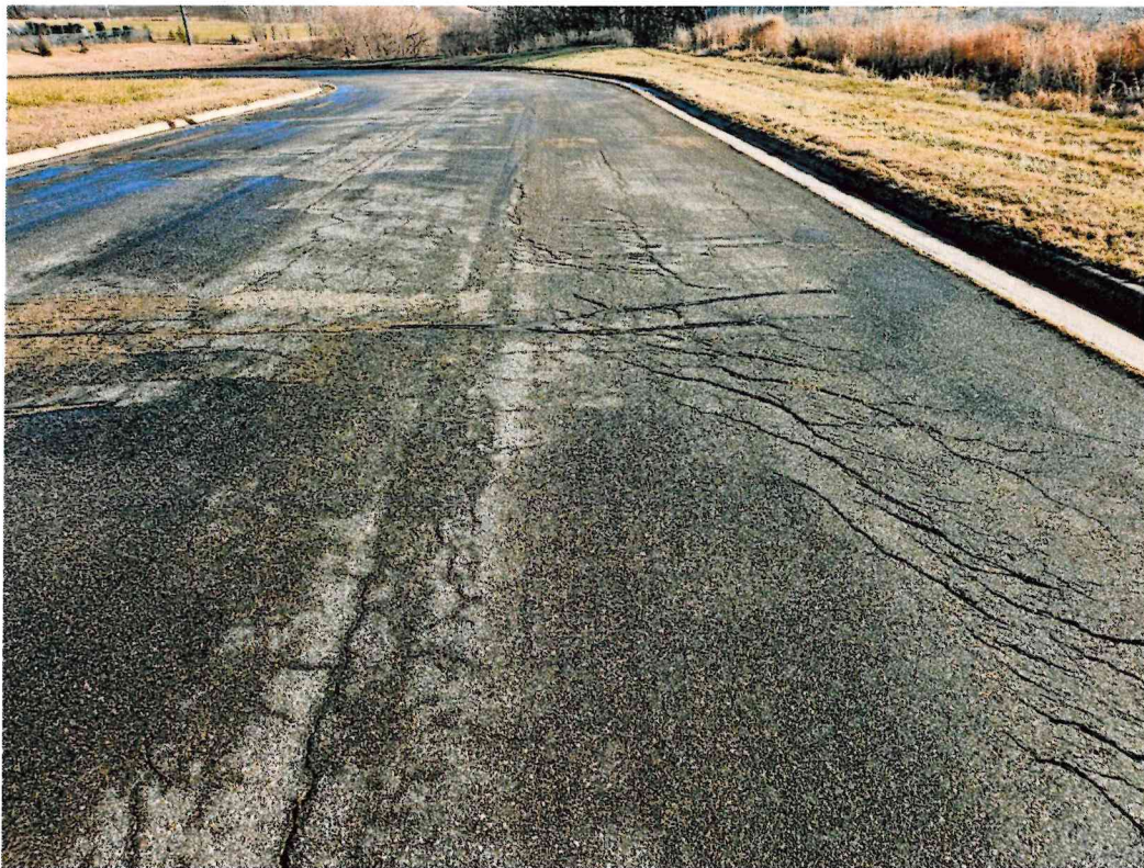
4 – Ross Drive – Deteriorated Pavement
