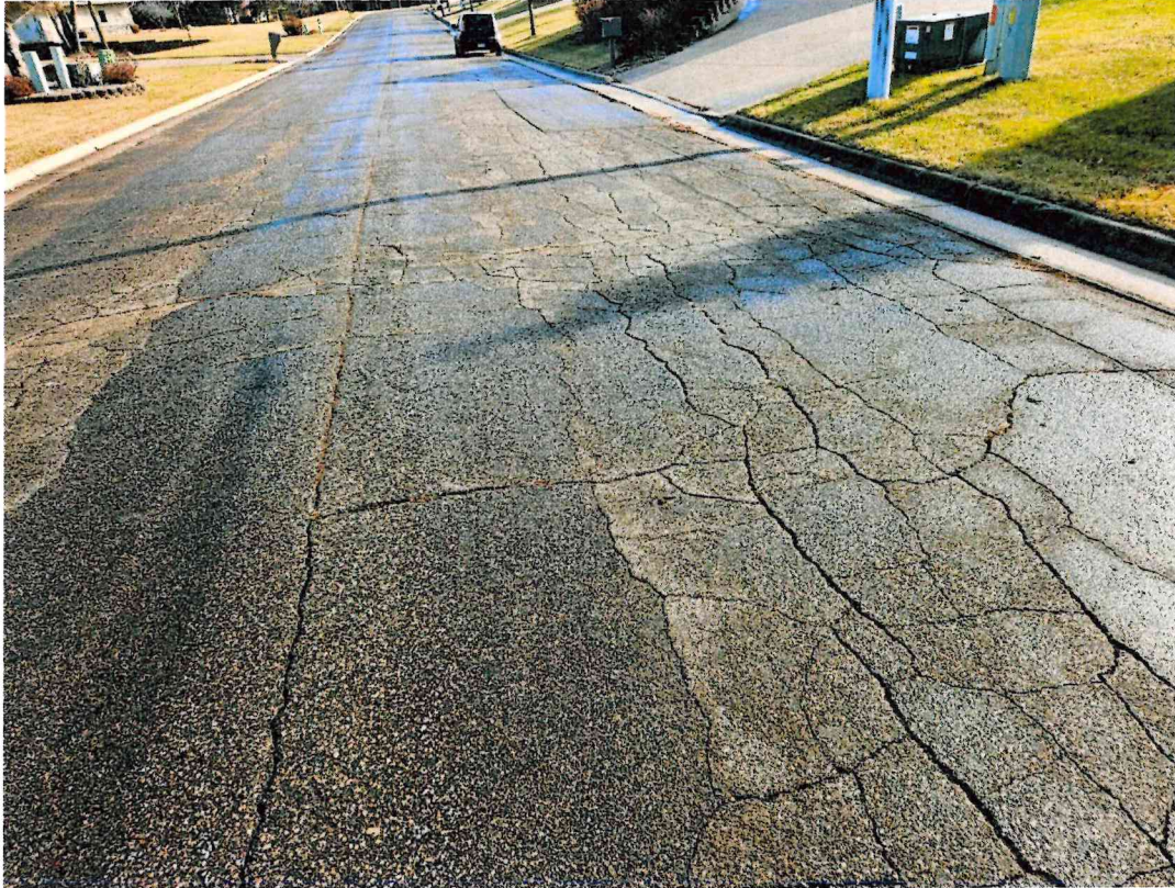
1 – Lake Chapeau Drive: Alligator Cracking
