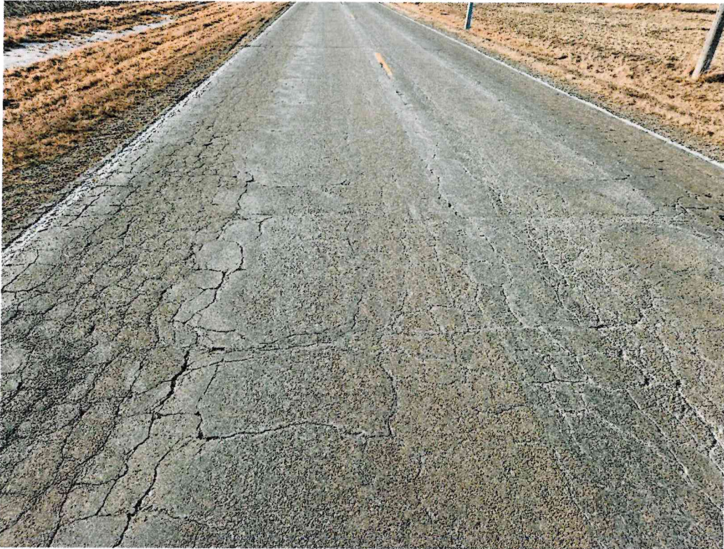
5 – SE Marshall St – Deteriorated Pavement
