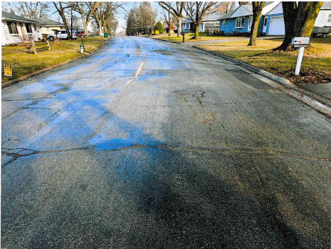
2 - Garfield Ave - Transverse & Longitudinal Cracking
