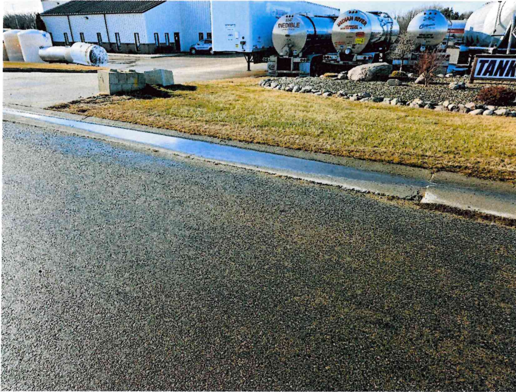
3 – Crossroads Blvd – Settled Curb
